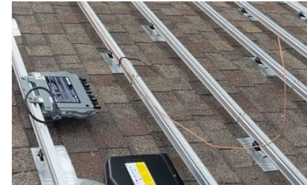
Mounting System Anchoring: Before modules are placed a photo showing the mounting systems anchoring technique utilized for applicable roof mounted projects must be captured.
